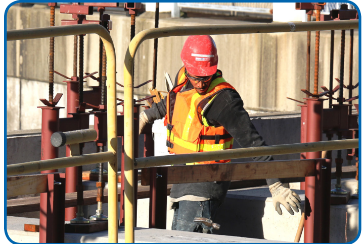
Marquies Patterson, a pre-apprenticeship graduate and Laborers apprentice, puts finishing touches on a newly installed section of seawall.
